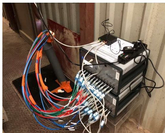
Figure 6: 2 PhosCapt-MP placed in Cell C, monitoring 23 lines with Ethernet remote control
